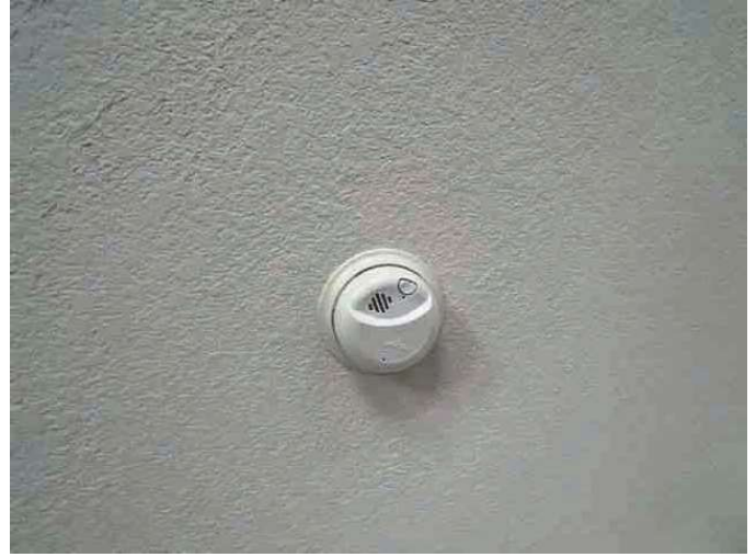
Smoke/Carbon Monoxide Detector
